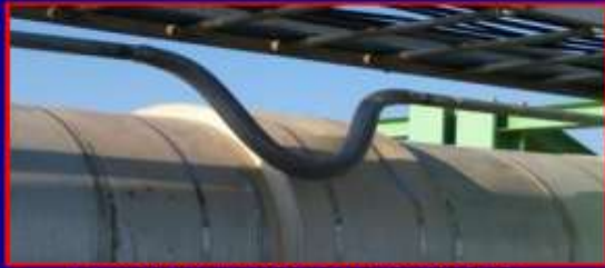
Bellow Leakage Collection Line
